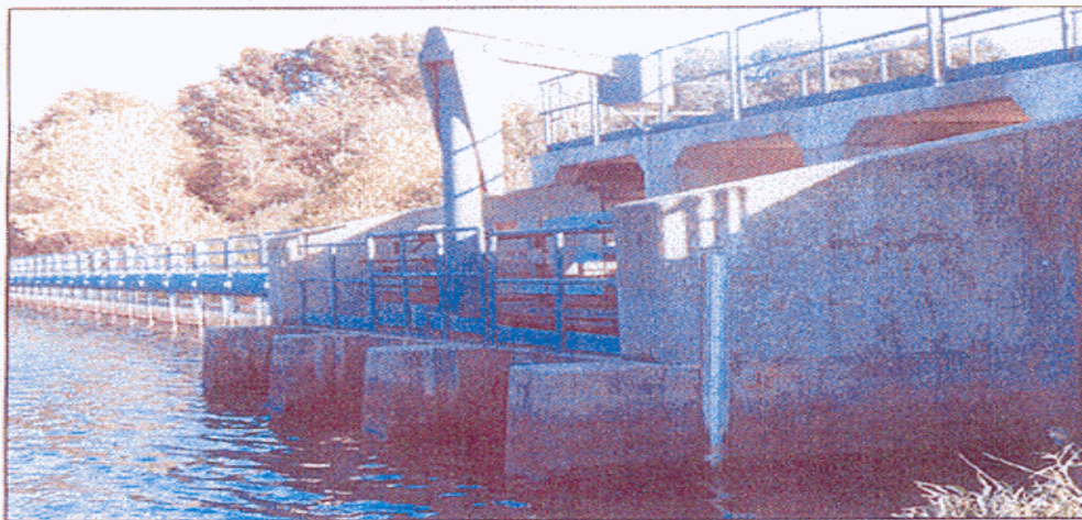
Photo 30 - Upstream view of outlet works control structure. Note reservoir staff gage mounted on wall.
