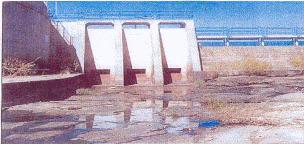
Photo 29 - View of outlet works control structure, looking upstream. Photo was taken prior to exercising gates, with no leaks through the gates.
