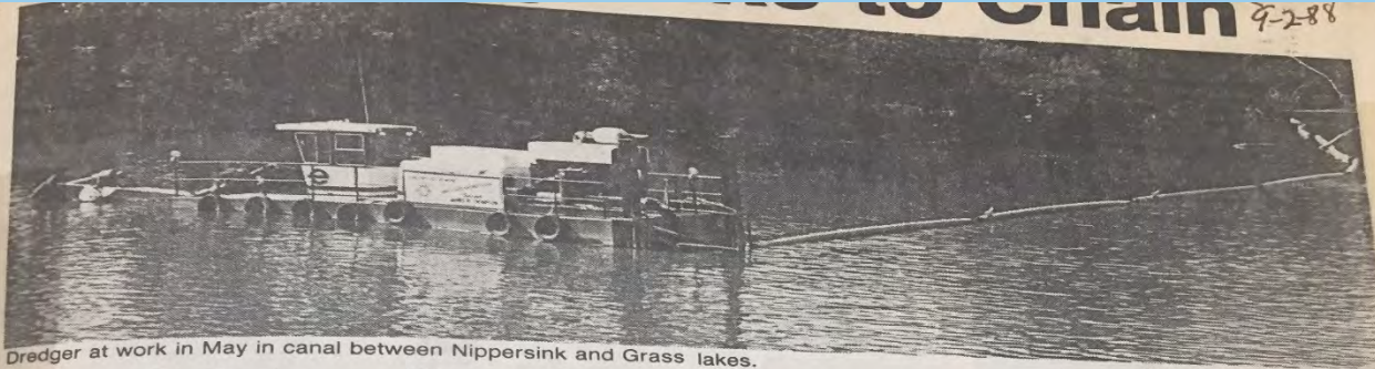
Dredger at work in May in canal between Nippersink and Grass lakes.
