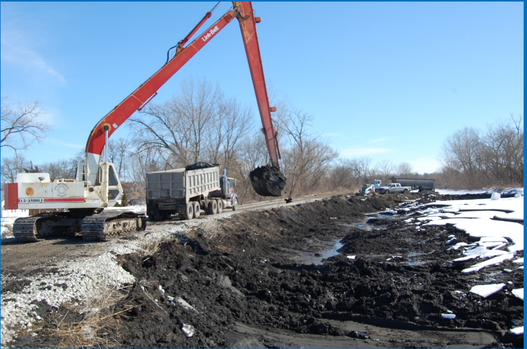
Fox Waterway Agency Drying Pond
